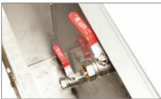
supply valve to fill a pit up and a drainage valve are situated in the front wall of the form
